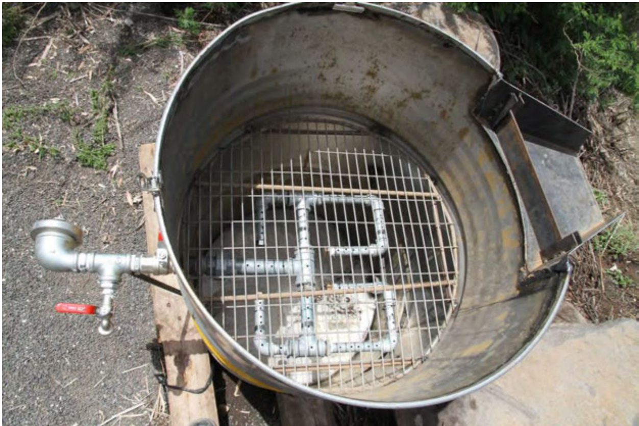
Figure 133, the floatation device is built using a barrel with a water distribution installation.
