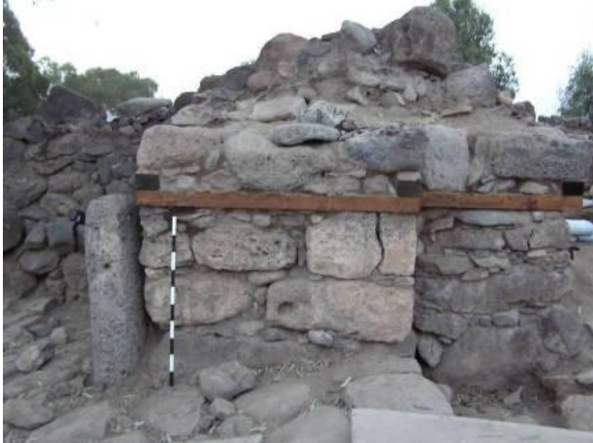
The southern door jamb at the inner gate, notice the wooden beams on top of three courses of stone.
